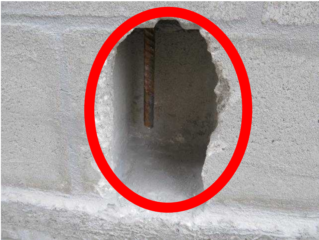
#6 Missing total of 4 footer dowels
