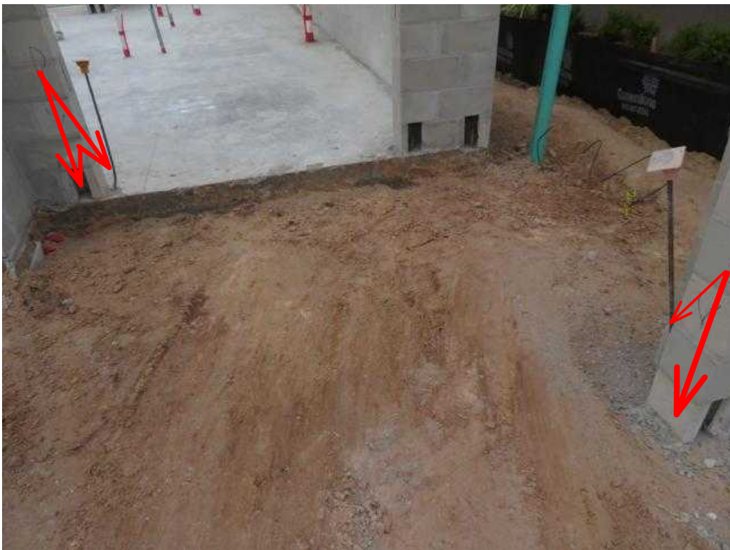
#18 Dowels placed improperly at slab pour at 2 places
