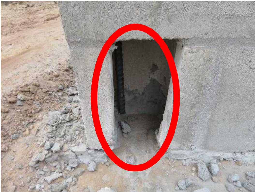
#20 Missing total of 4 footer dowels
