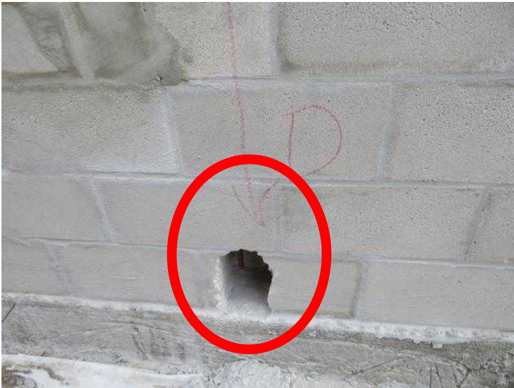
#4 Missing total of 4 footer dowels
