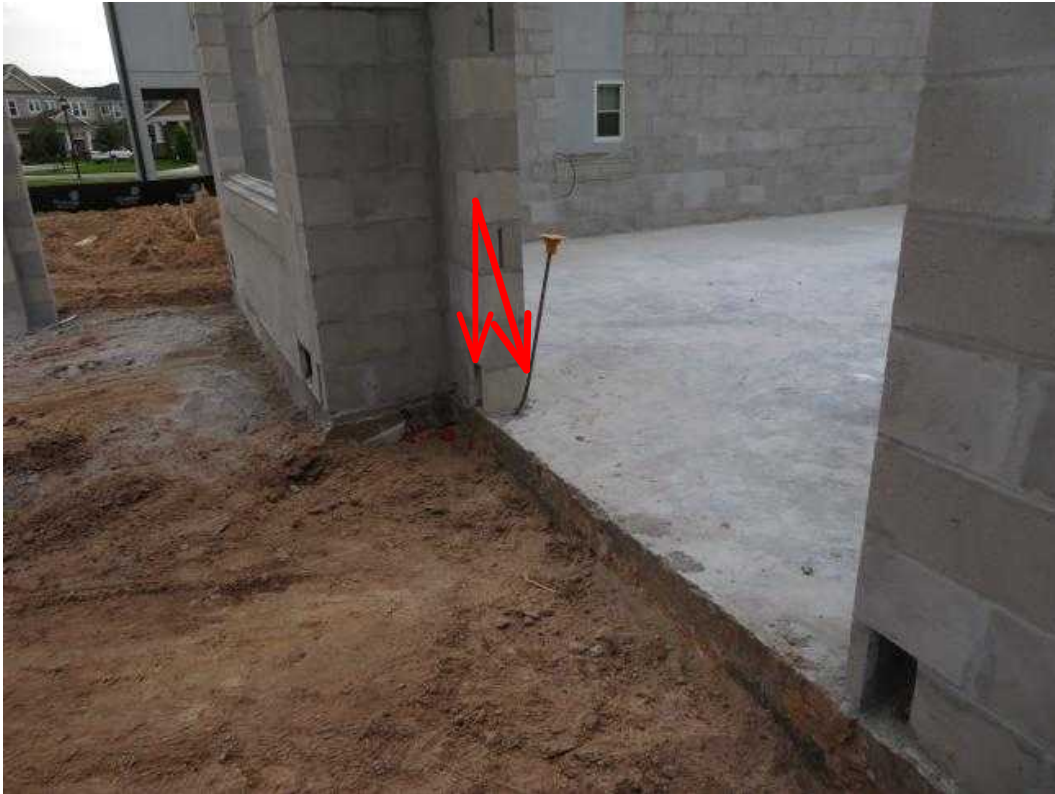
#15 Dowels placed improperly at slab pour at 2 places
