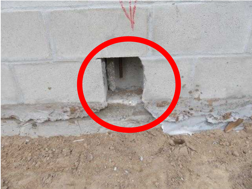
#3 Missing total of 4 footer dowels
