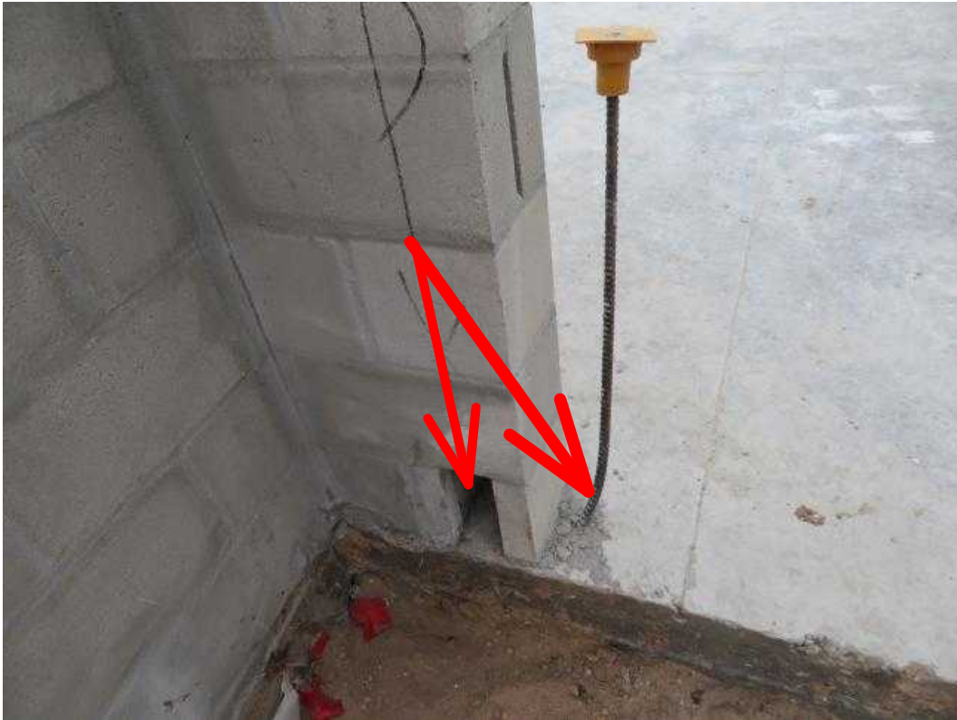
#13 Dowels placed improperly at slab pour at 2 places
