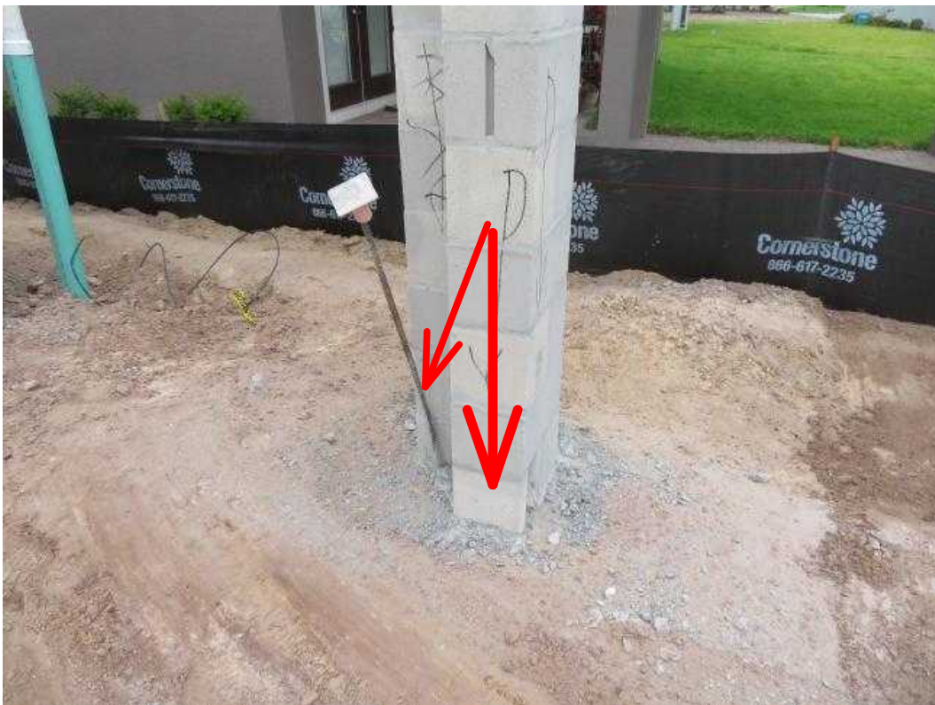
#16 Dowels placed improperly at slab pour at 2 places
