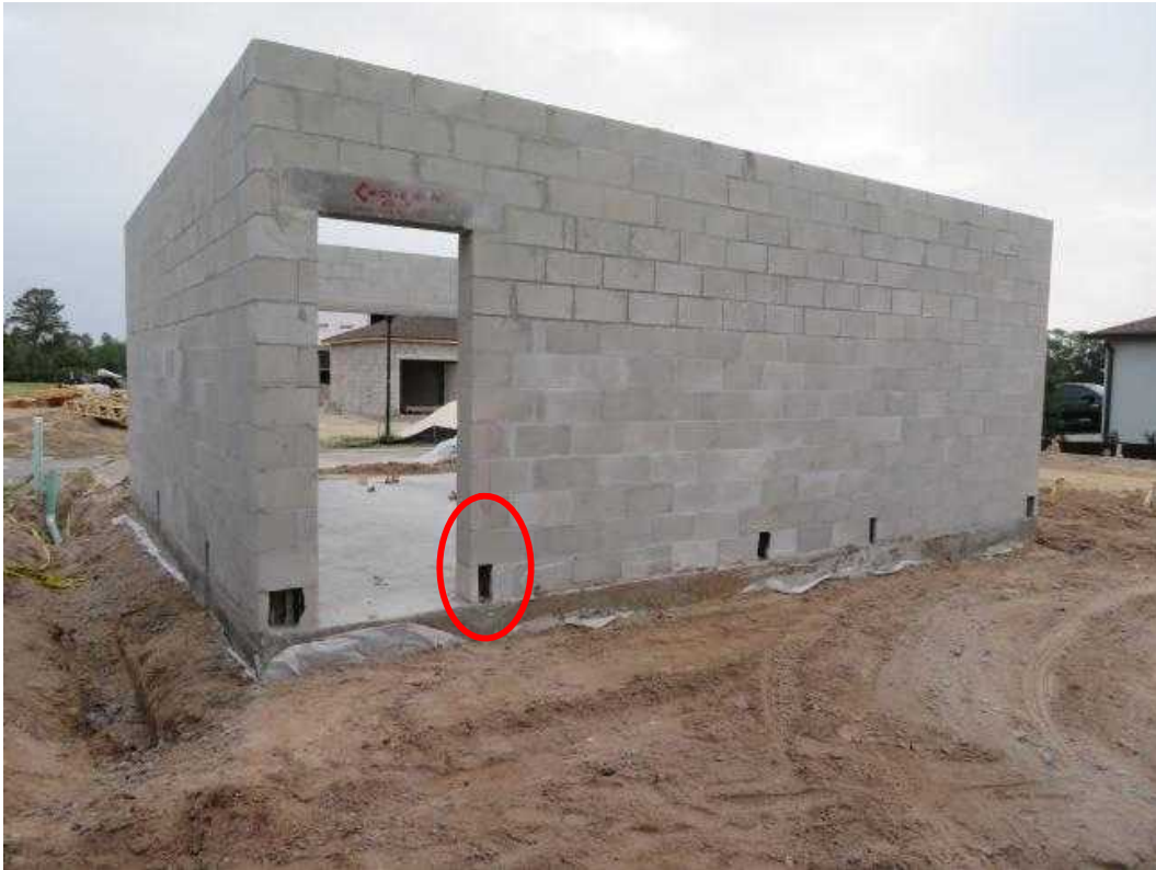
#23 Missing footer dowel at garage
