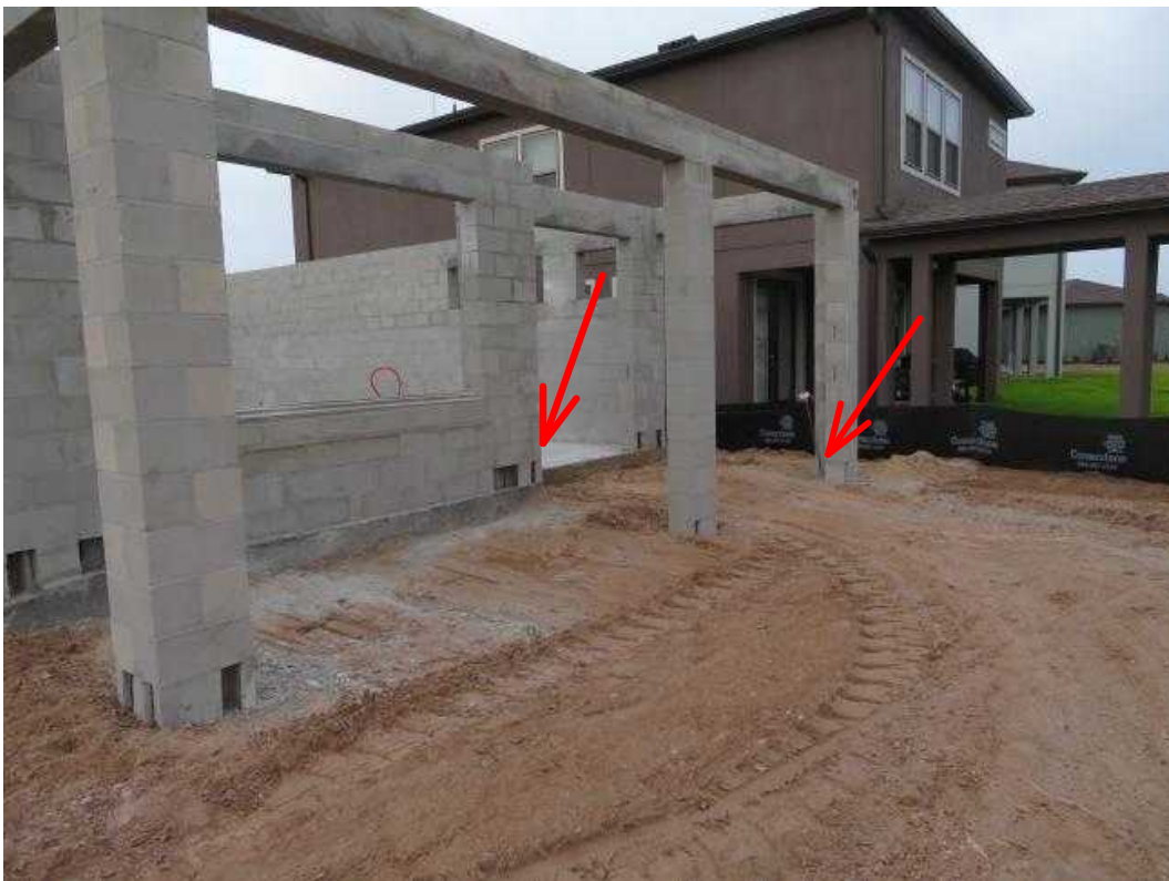
#14 Dowels placed improperly at slab pour at 2 places
