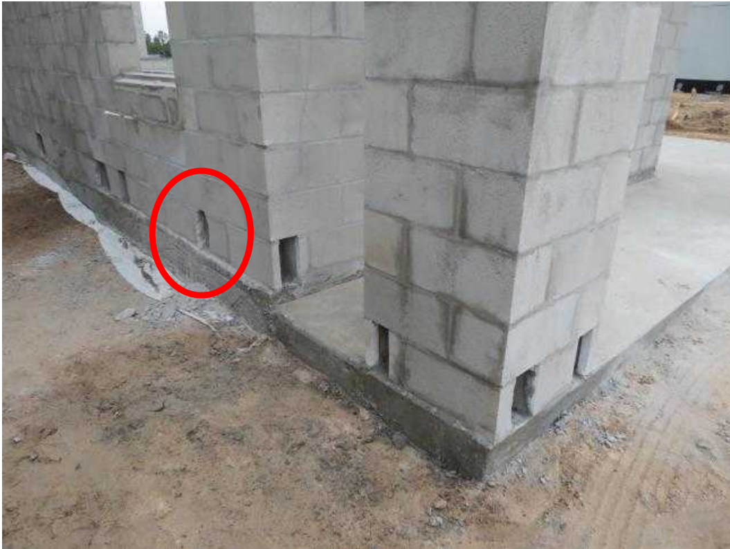
#5 Missing total of 4 footer dowels
