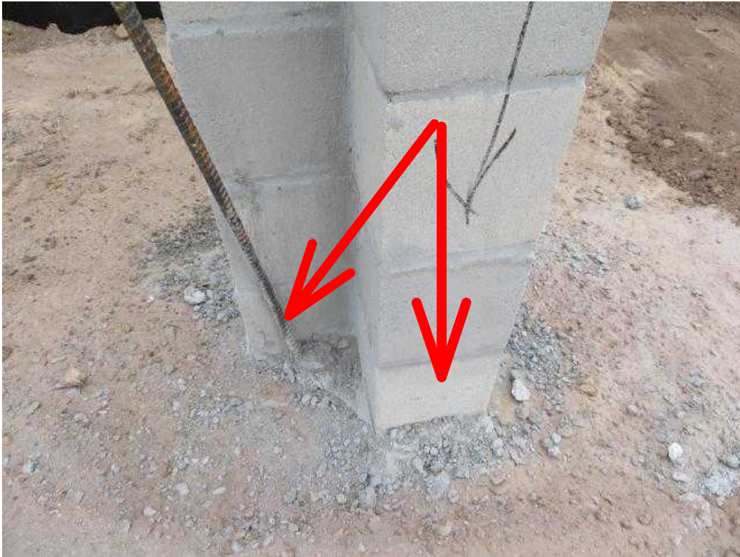
#17 Dowels placed improperly at slab pour at 2 places
