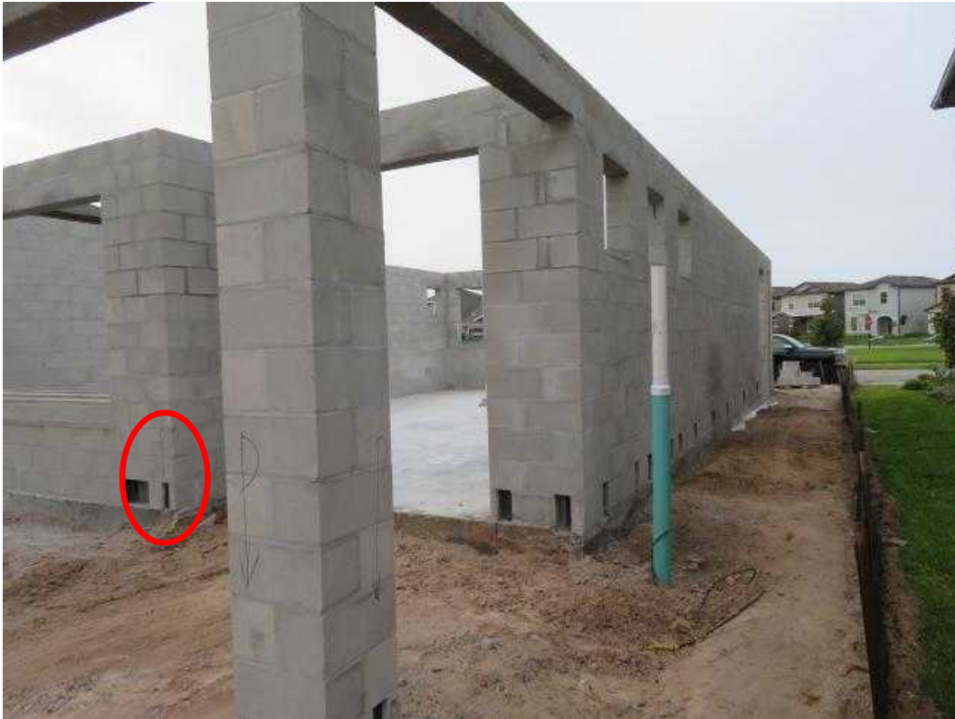
#21 Missing total of 4 footer dowels
