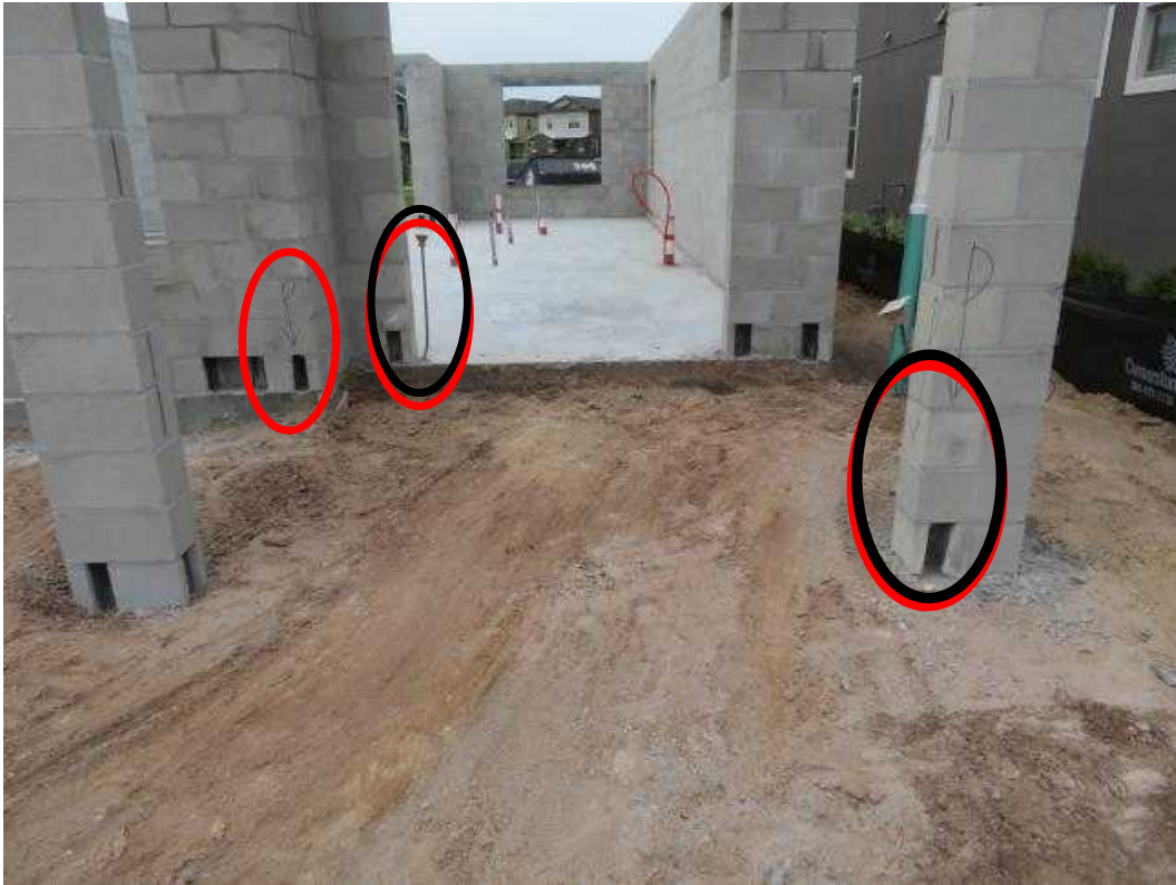
#9 Black: dowels placed improperly. Red: missing footer dowels
