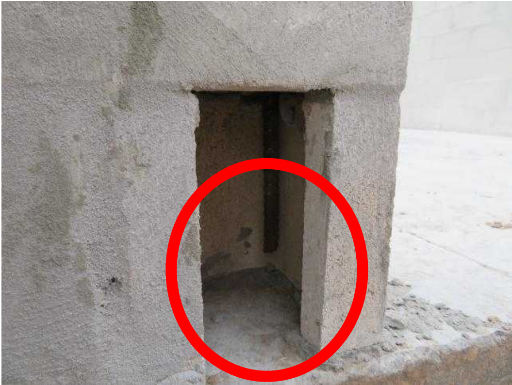
#19 Footer dowel missing. All dowels were present at footer inspection
