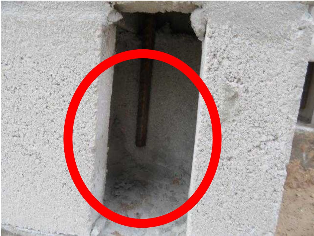
#7 Missing total of 4 footer dowels
