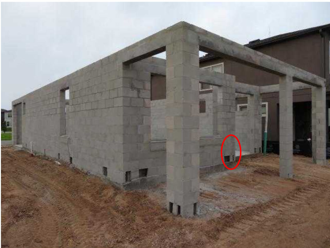
#22 Missing total of 4 footer dowels
